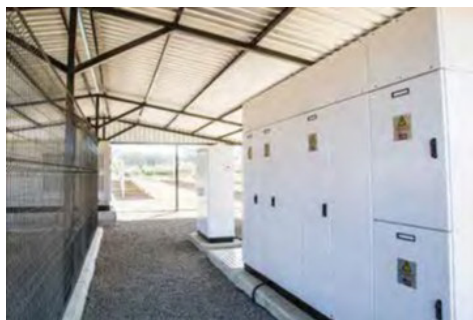
Figure 4: Having a state-of-the-art solar system has guaranteed the farm fixed energy costs for the next 25 plus years
