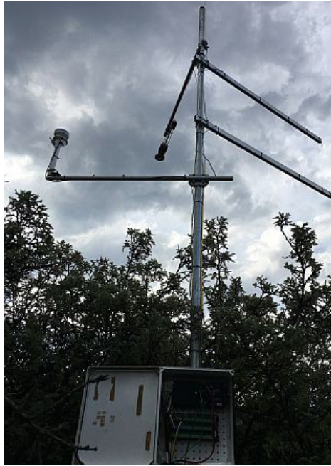
Figure 4: The fully installed Surface Renewal system in the woody encroached Catchment IX
